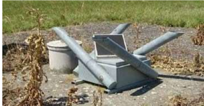
Figure 6- An underground stationary gas powered noise generator
