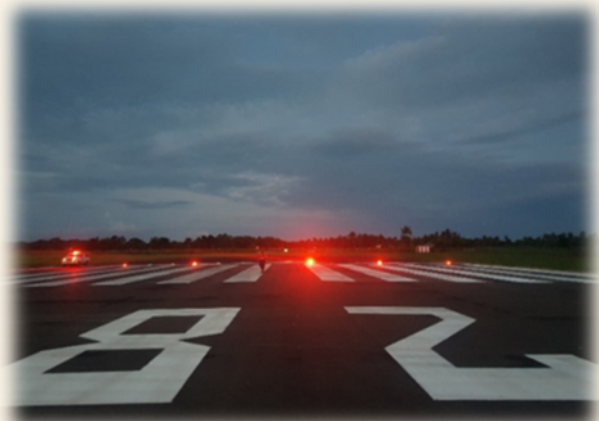
Figure 6 - Nausori Airport Runway 28 End Identifier Lights
